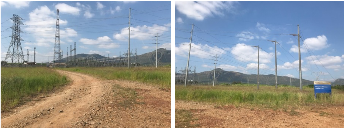
Figure 10: View from the gravel road towards the Khanyazwe substation
